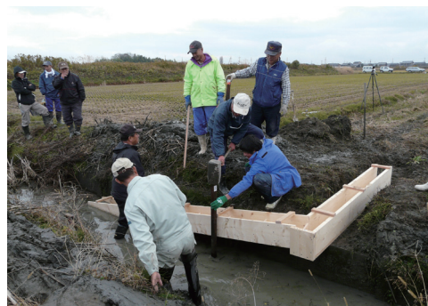
(photo 3) Setting small-scale fish-ladder (Chidori-Xtype tuned in TAKASHIMA), which is fit to the water level management of pesticide free organic farming method.
